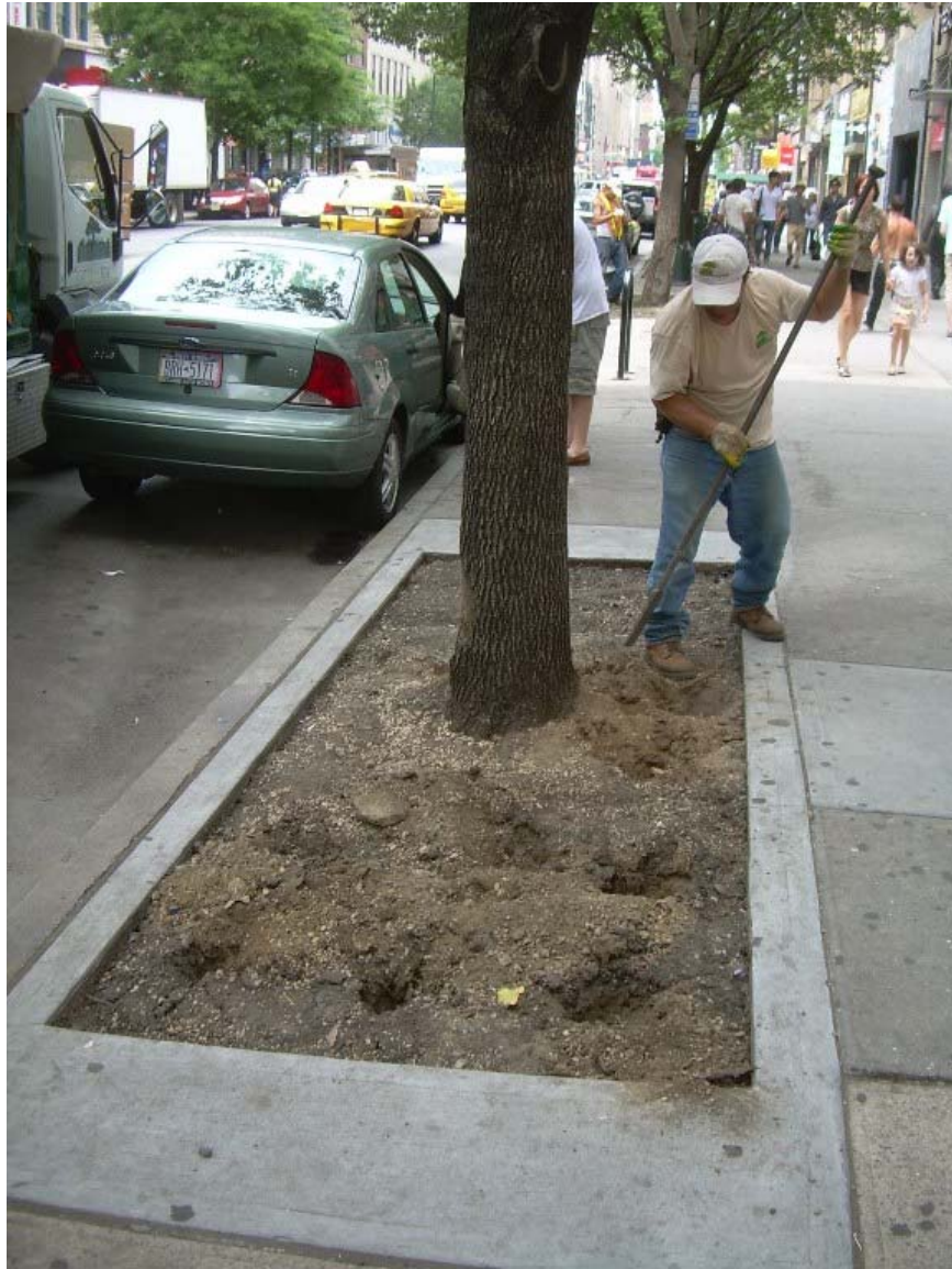
5. Once the saddles were removed, Urban Arborists was hired to aerate the soil, which had compacted tightly after almost 20 years under the weight of the metal grates.
